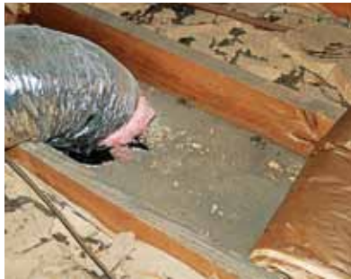
This photo was taken in the home of Marla Eversole. Note the way the insulation is rolled away from ducting, leaving no insulation in that area!
