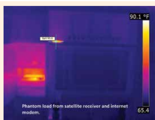
The infrared picture shows where hot spots are located; in this instance heat is coming off the satellite receiver and the Internet modem. This represents electricity in use or Phantom load.
